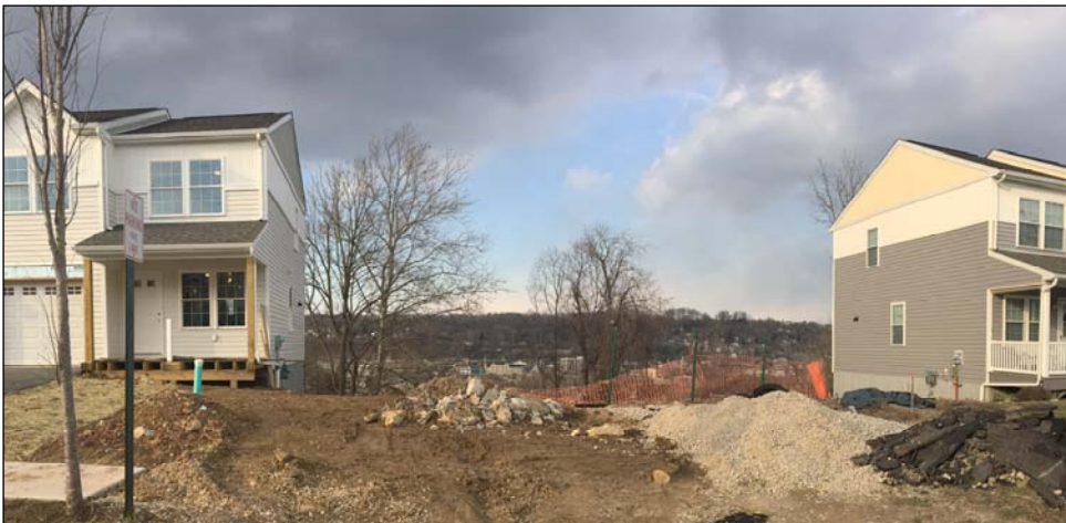
The future site of the next Habitat home. This will be the last home on this side of the street.
